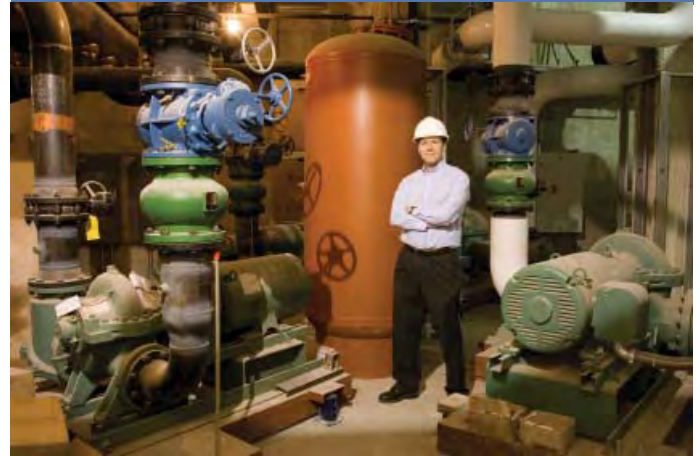
Maintenance Review - Engineer inspecting existing conditions and efficiency of hydronic systems.
