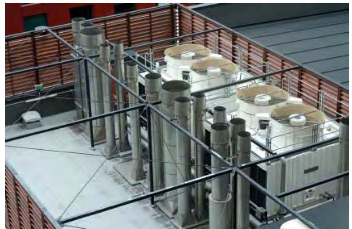
Fume Hood Exhaust - Pictured are lab fume hood exhausts and process cooling towers.
